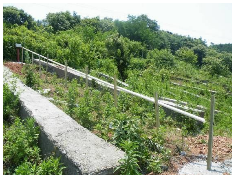
图 4 现场安装图 Fig.4 Photo of field installation
